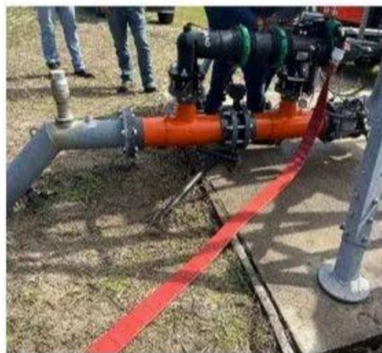
(F) Filtration System
