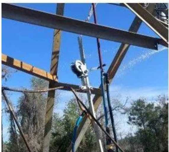
(E) Winch system at the end of the pivot
