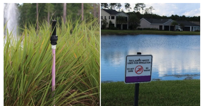
Figure 2. All reclaimed water piping, fixtures, valves, heads, etc., are required to be purple in color and labeled “Do not drink this water.” Credit: Terra Freeman, UF/IFAS
