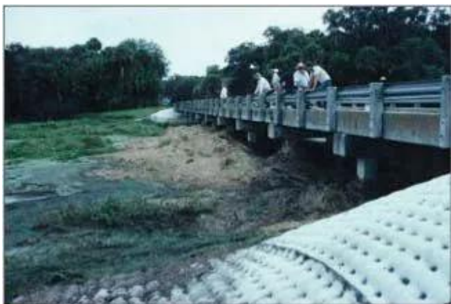
Figure 16. Submersed plants piling up on a bridge in South Florida.
