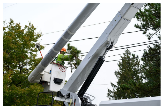
Figure 4. Only qualified line-clearance arborists can work on trees near power lines such as with this aerial lift.
