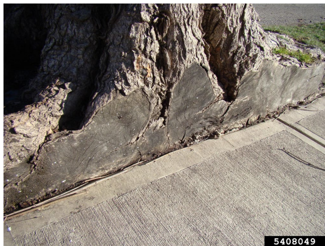
Figure 18. These tree roots were severed during sidewalk and curb repair, making them prone to toppling during a hurricane.
