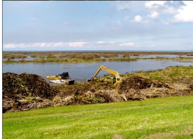
Figure 24. Mechanical removal by operating a harvester with removal belt (top) and by pushing weeds on shore for harvesting with a track hoe (bottom).
