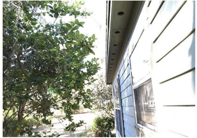
Figure 6. Branches cut away from roof and walls so that pests cannot use them to access home.
