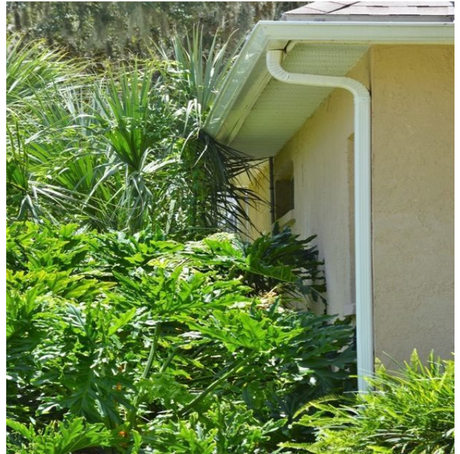
Figure 7. Overgrown plants allowing access to the roof.
