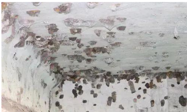
Figure 17. The underside of a bridge in north-central Florida with a high density of Sceliphron caementarium (Drury) mud nests.
