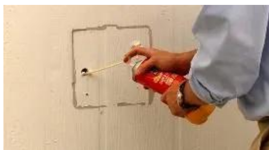
Figure 21. Foaming holes inside of a building.
