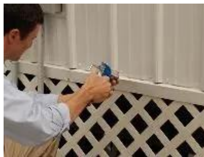
Figure 20. Caulking opening in siding.
