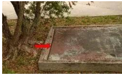
Figure 5. Open space in metal drain cover.
