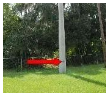
Figure 17. Small hole in power pole.
