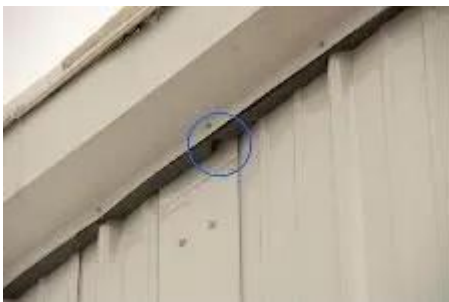
Figure 3. Small hole in siding leading to a cavity in the wall.
