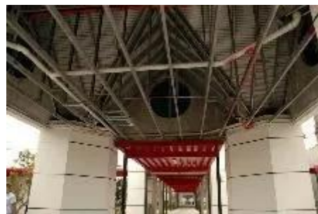
Figure 7. Large recess under roof.
