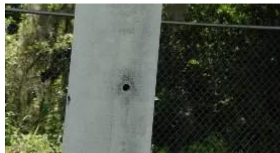
Figure 16. Small hole in power pole.
