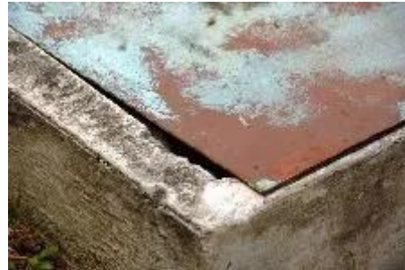
Figure 6. Crack in cement that creates opening.
