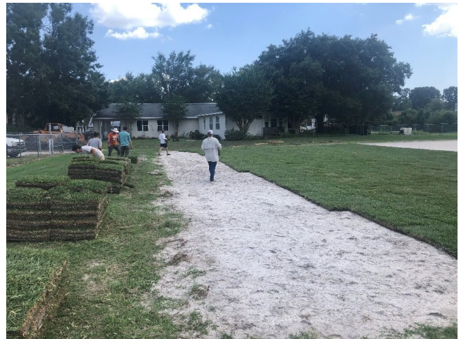
Figure 1. Sodding produces an instant ground cover. Lay sod pieces in a staggered pattern so that the seams are offset between pieces.
