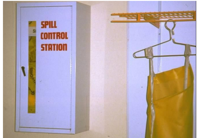
Figure 1. Permanent-sited spill kit cabinet. Credit: UF/IFAS
