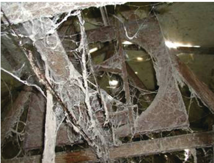
Figure 3. Broken fans and buildup of dust. Credits: UF/IFAS
